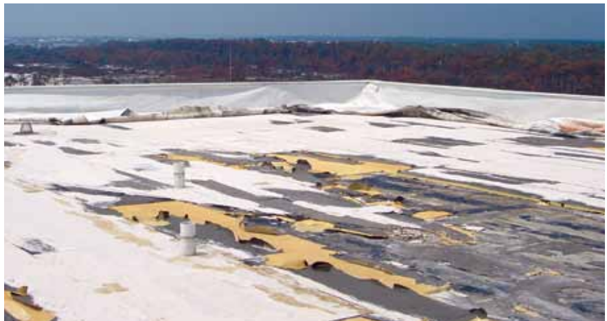
Hurricane wind literally peels single ply membrane from roof deck.
