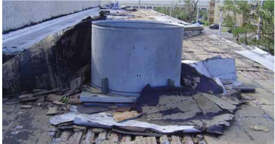
Asphalt membrane roof failed due to high winds even though fasteners remain attached.
