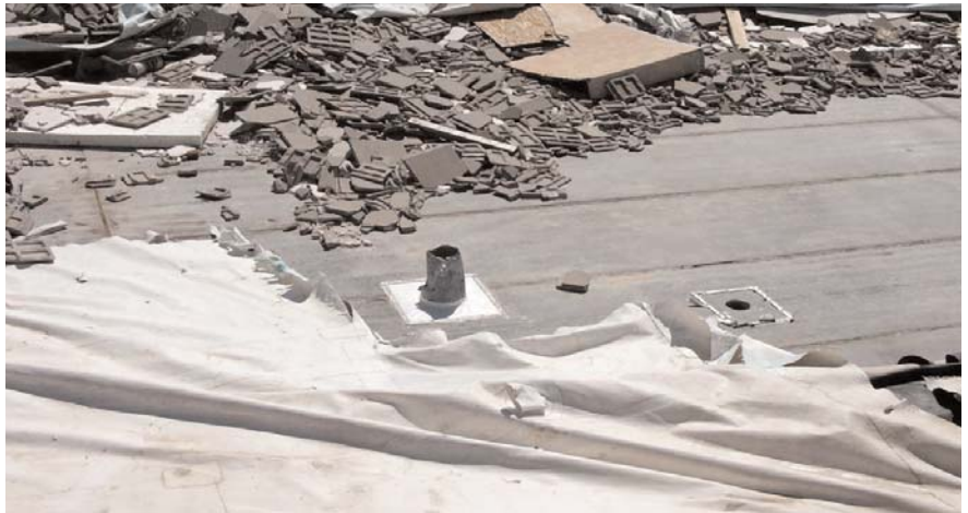
Concrete paver – ballasted TPO membrane roof system destroyed by Hurricane Ivan.
